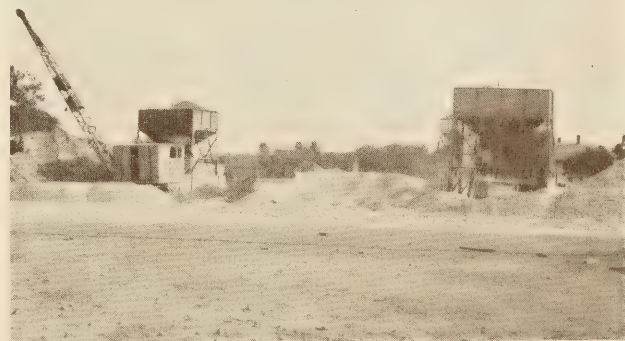
FIGURE 8.—TYPICAL PLANT SET-UP USED ON STATE-AID PROJECT 2926, SHEBOYGAN COUNTY, WIS. MATERIALS HAULED IN BY TRUCK FROM A LOCAL PIT. COARSE AGGREGATE SEPARATED IN THREE SIZES
